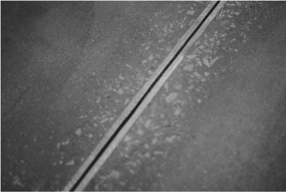
Figure 15.8 This armoured joint (flat-bar type) needed grinding
