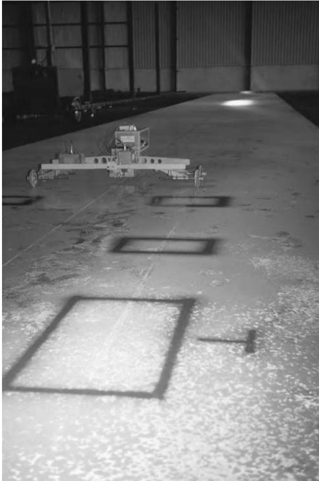
Figure 19.9 Superflat construction – marking a new slab for grinding, after testing with a profileograph
